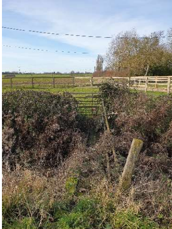
Figure 1, FP9. Bridge rotted and path blocked by fencing.
